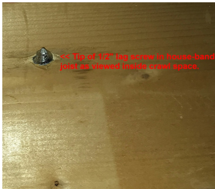
Figure 6. The visible tip of the lag screw as depicted indicates compliance with the IRC requirement that lag screws fully extend beyond the inside face of the house floor band joist. (Photo by Frank Woeste)
