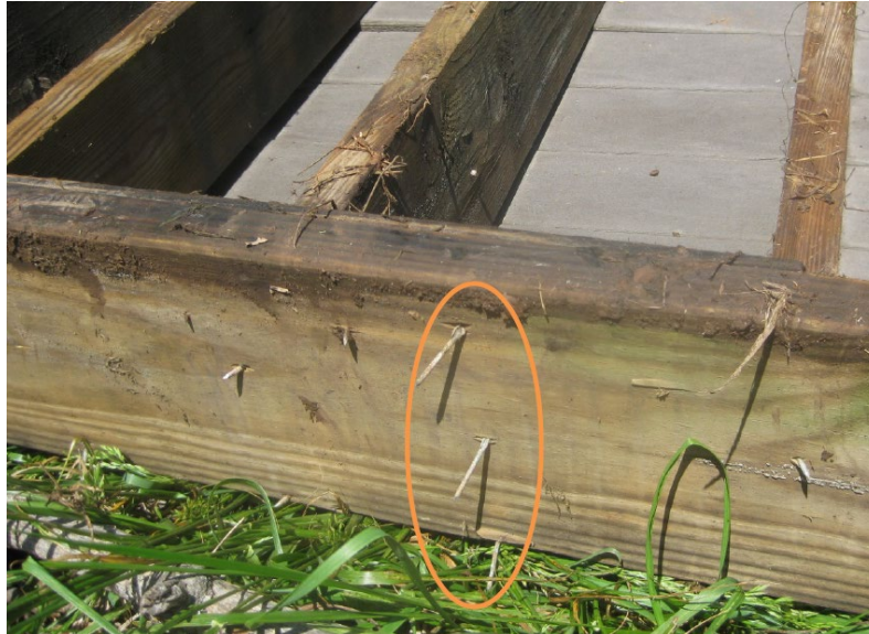
Figure 3. Close-up of deck ledger that was connected to a structure with nails only. Even though only lightly loaded by occupants, the deck shifted laterally, pulling the nails out of the supporting structure. (photo by Frank Woeste)
