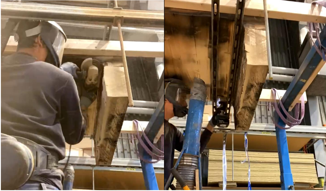
Figure 8: Using an angle grinder with a flap sanding disc to reduce the corner rounding (left) to allow the router on the planing frame to come as close to the corner as possible (right).
