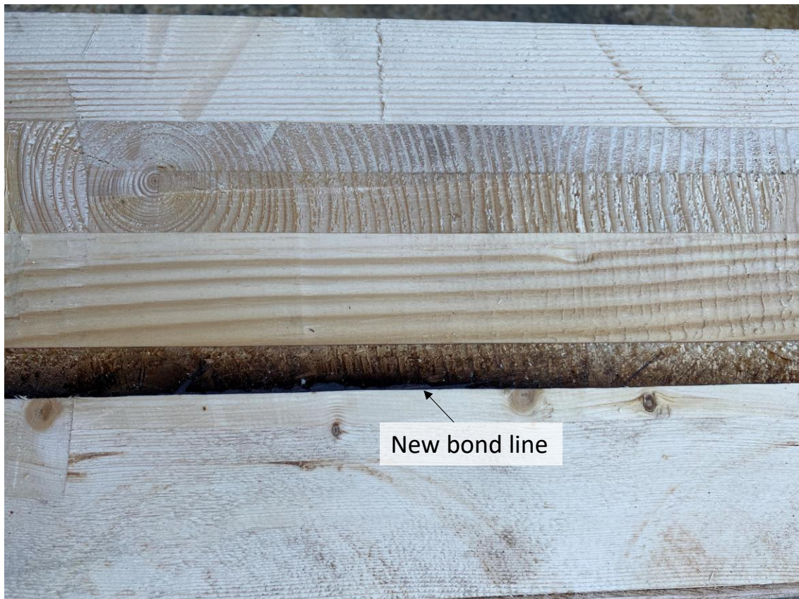
Figure 26: Photo of the longitudinal-section of the rehabilitated CLT member at the location where the char depth slightly exceeds the milled depth.
