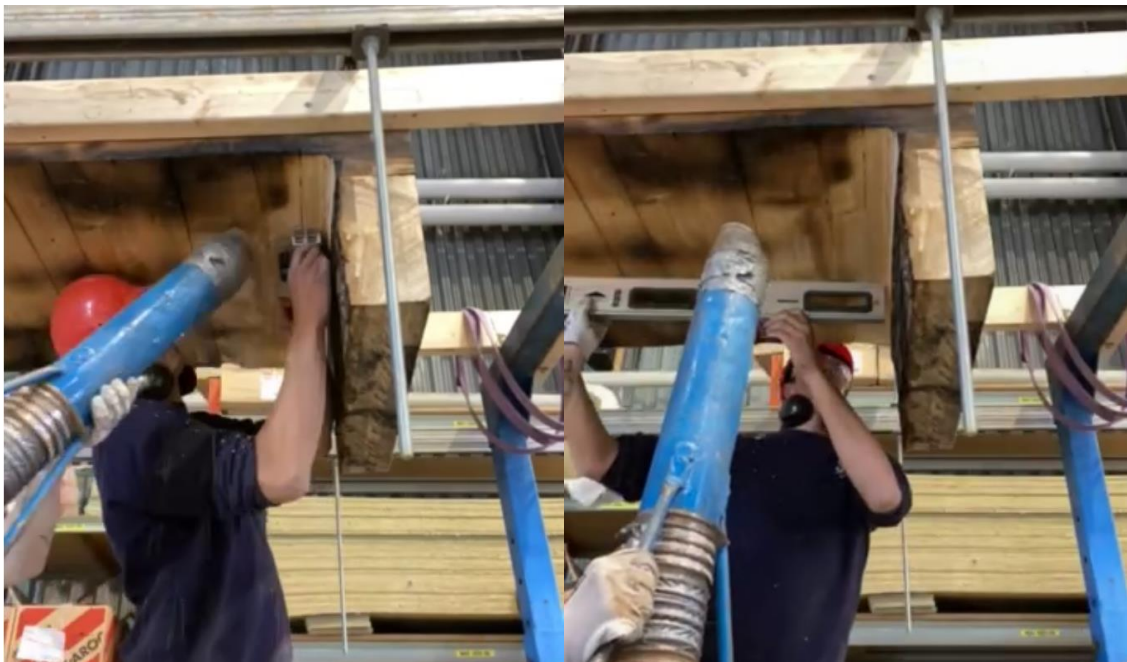
Figure 9: Using a planer specialised in planing near inner corners (left) and assessing the planeness of the surface (right).
