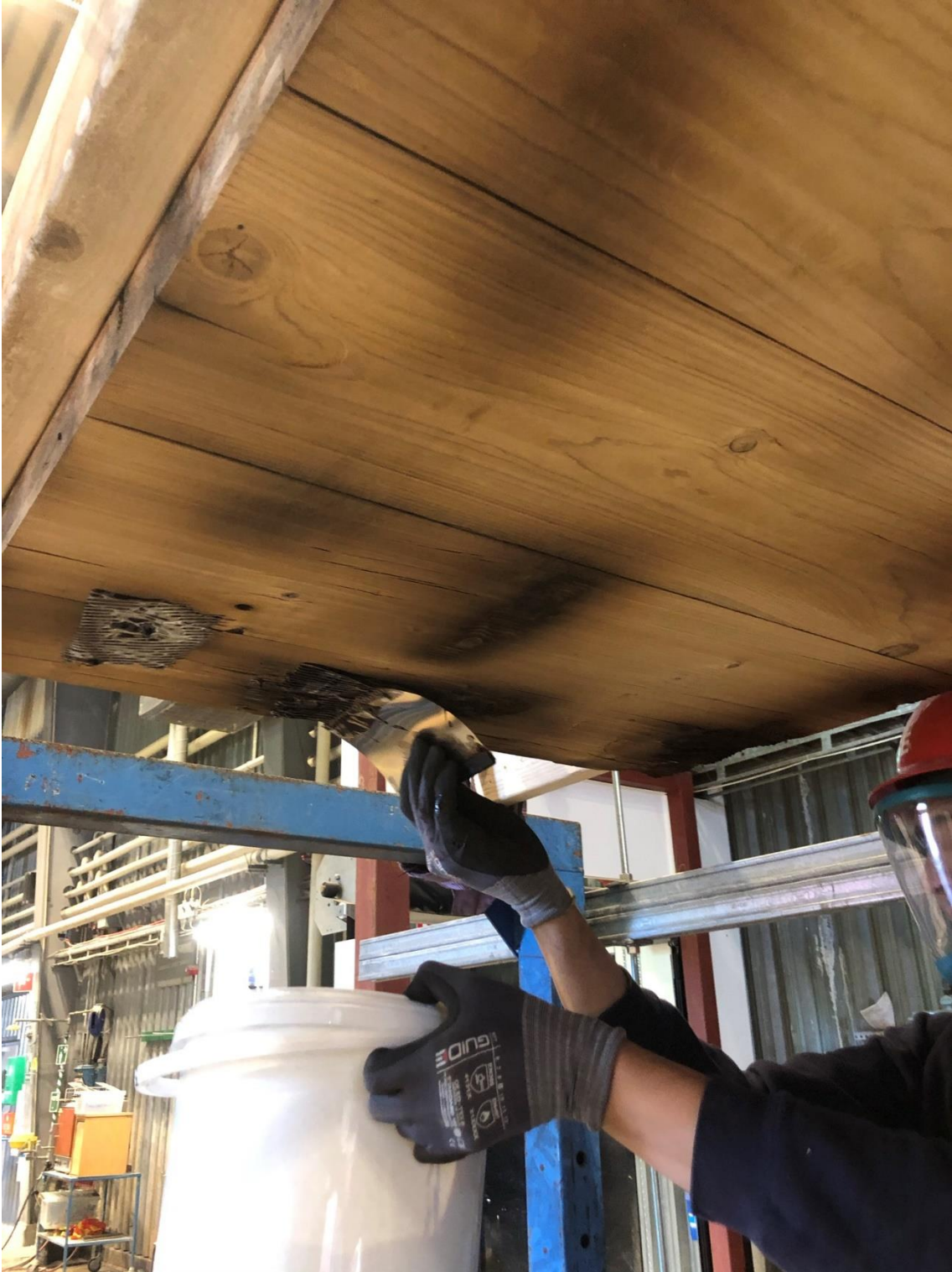
Figure 17: Applying adhesive on the ceiling with a glue comb at the locations in the ceiling with deeper char depths than the milled depth
