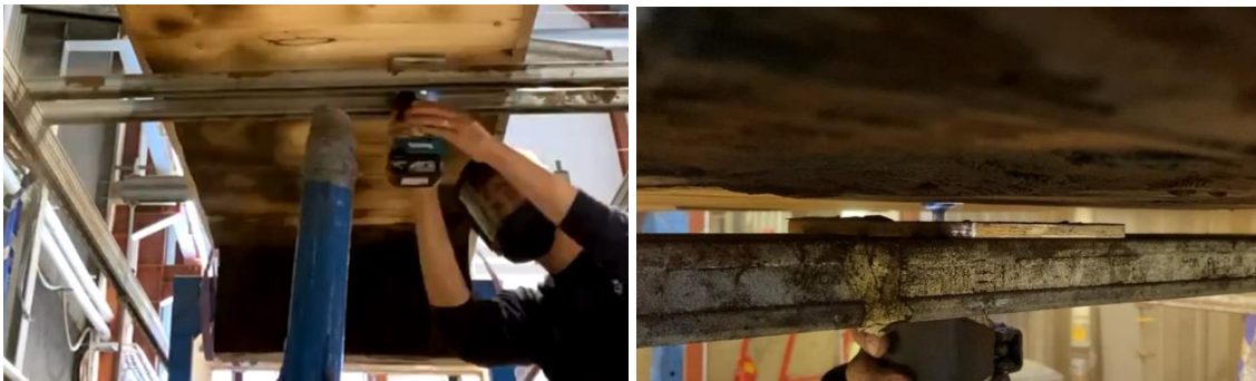
Figure 7: Planing of the charred surface with a router sliding on a frame (left and right)
