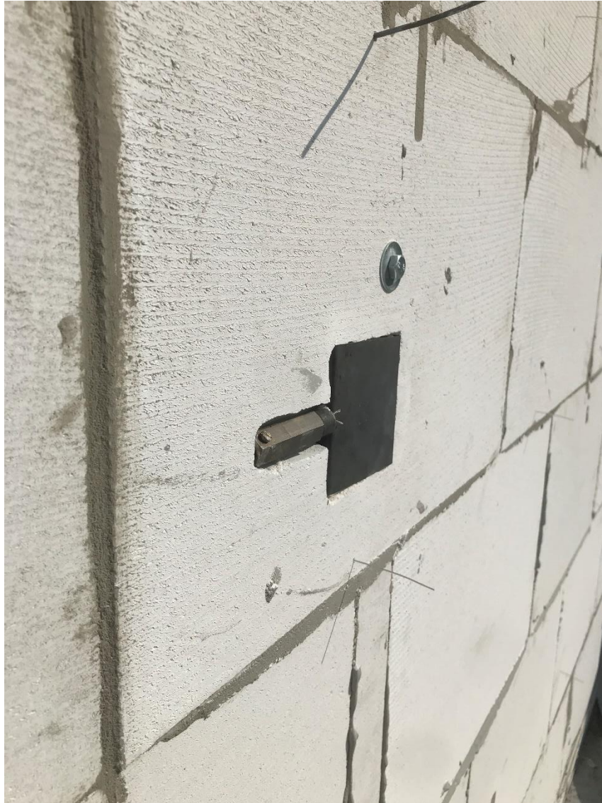
Figure 7. PT 4 embedded flush to the façade surface. Under the PT a 1 mm diameter TC (TC 7) extrudes 5 cm and above a 3 mm diameter TC extrudes 10 cm.
