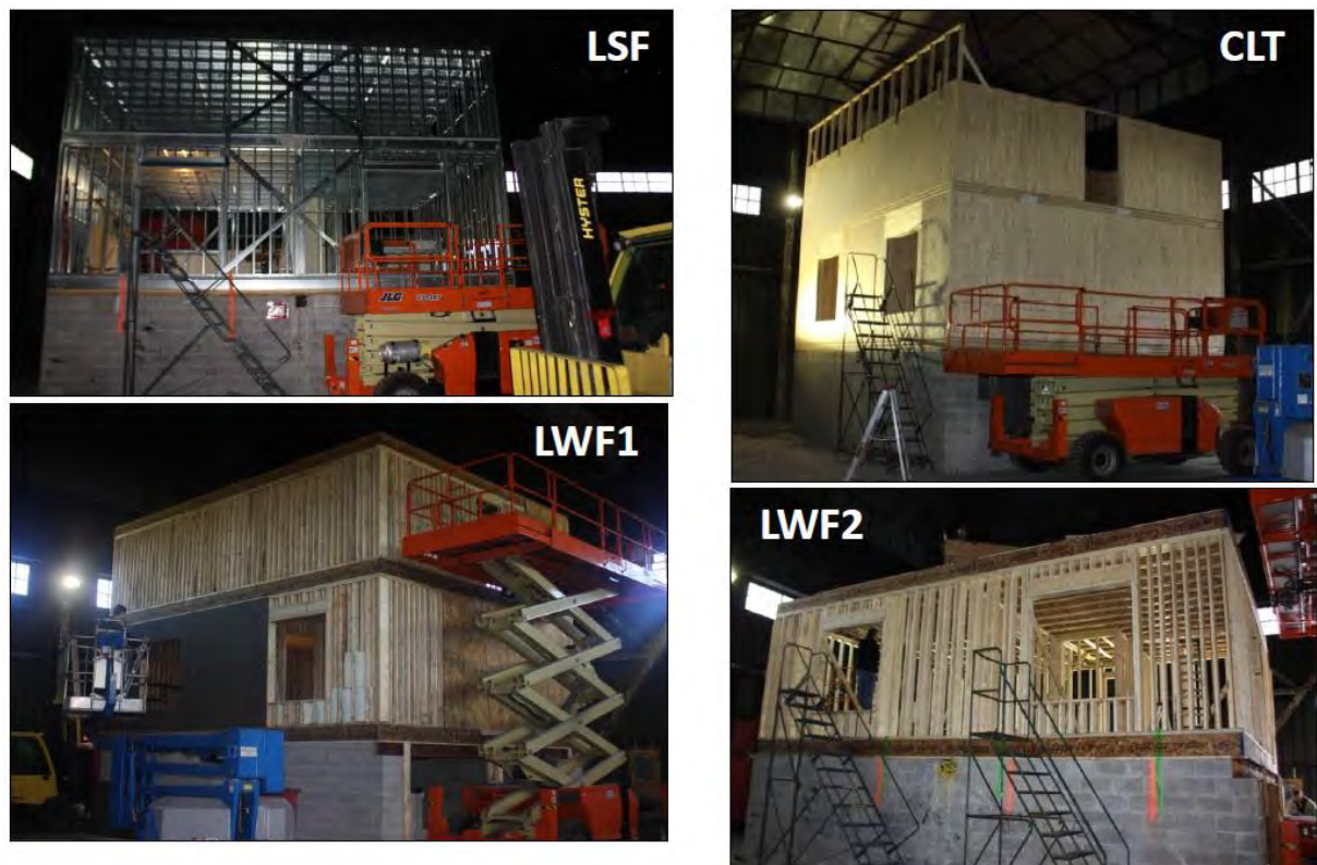
Figure 14: Compartments of test L1 (LWF1), L2 (CLT), L3 (LSF) and L4 (LWF2) under construction, from Su and Lougheed (2014)
