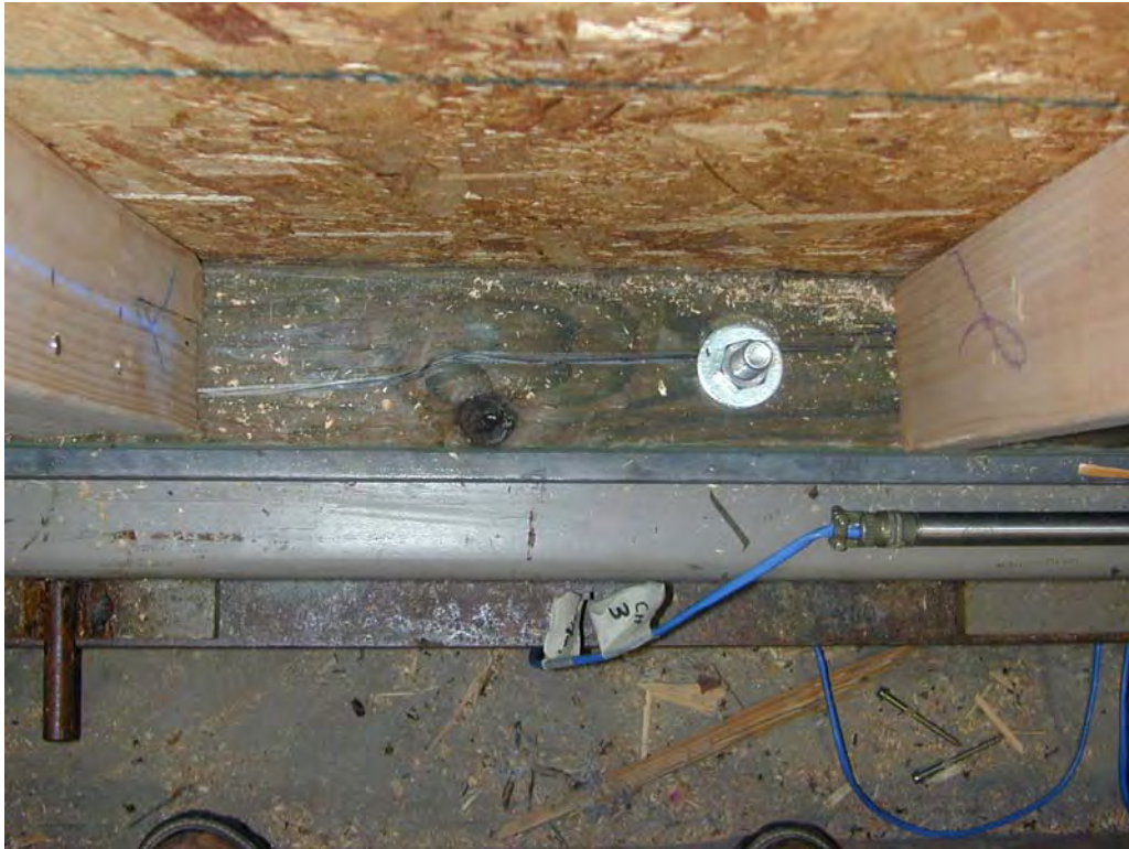
Figure 24. Sole plate split between interior studs (Specimen C1)
