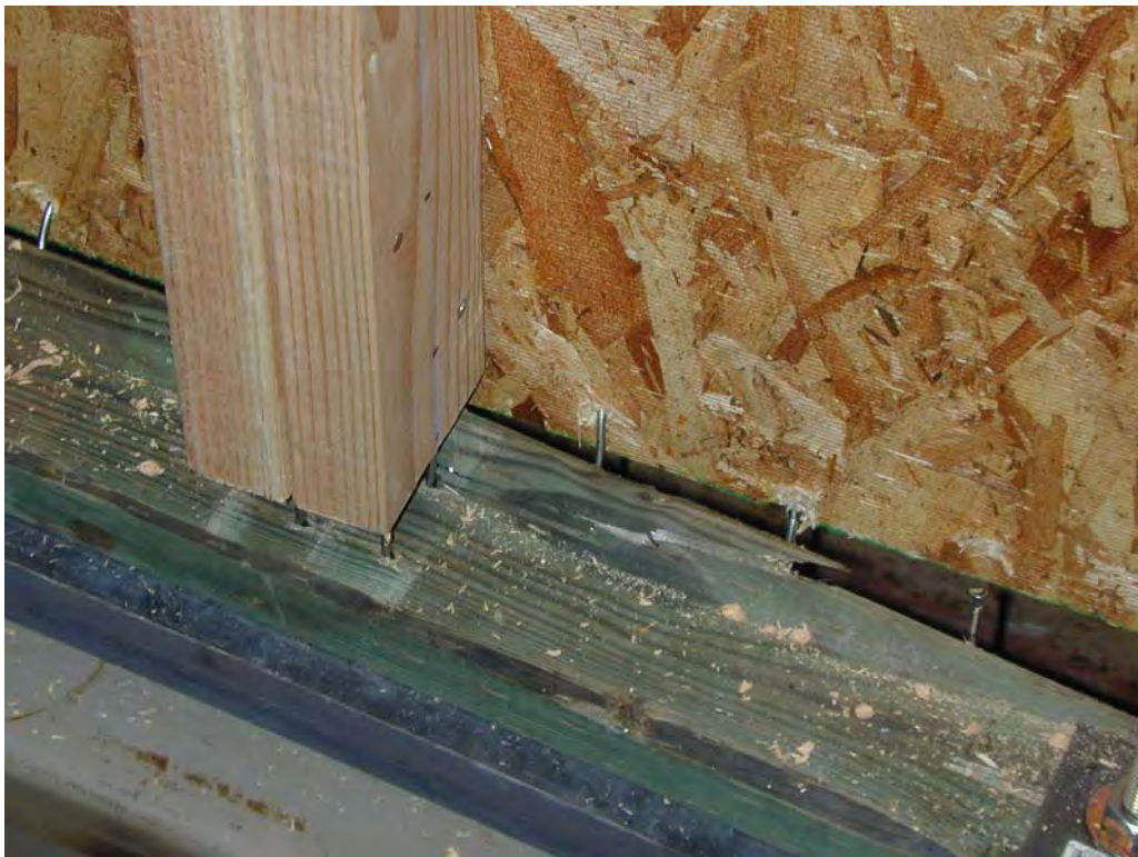
Figure 11. Failure at bottom of wall, some splitting of sole plate (Specimen A3)
