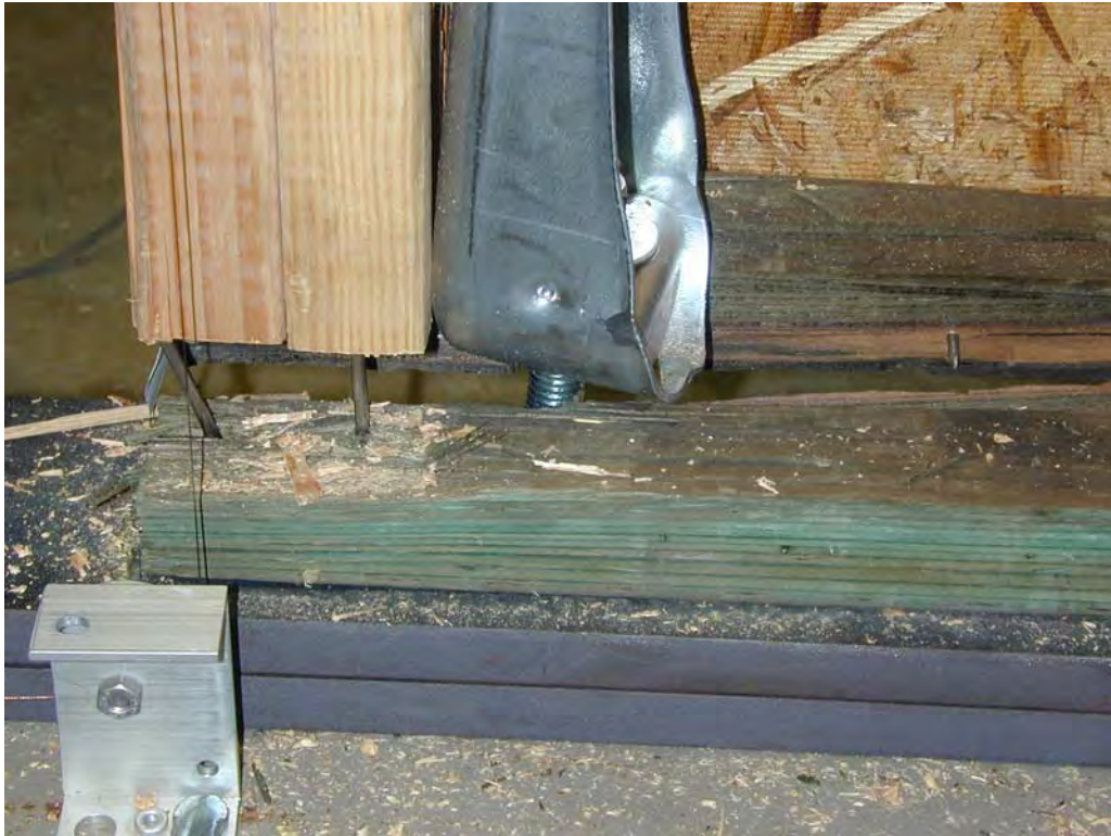
Figure 18. Sole plate splitting at hold-down (Specimen C1)
