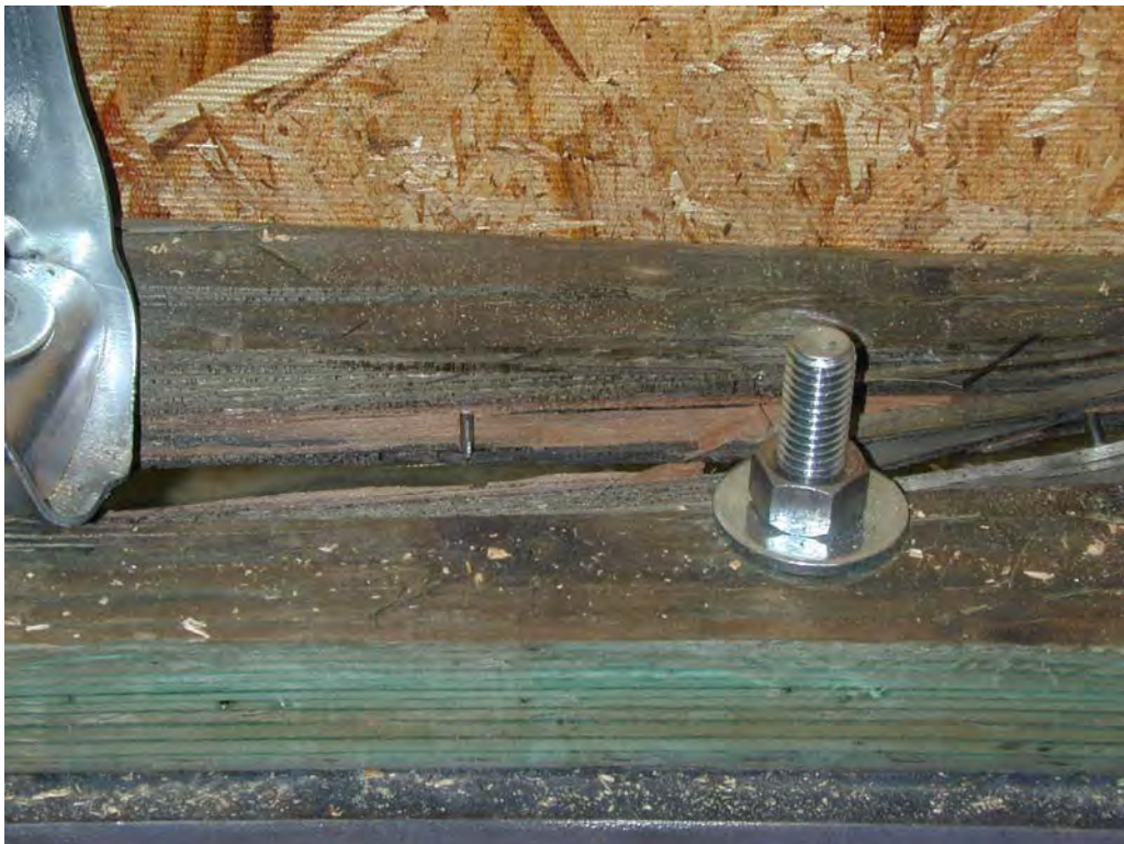
Figure 19. Sole plate splitting from hold-down to first washer location; no bending of washer (Specimen C1)
