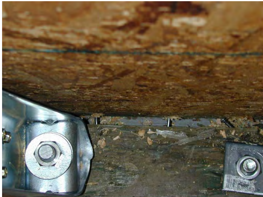
Figure 31. Sheathing separation from bottom plate, showing bolted anchor and hold-down (Specimen D3)
