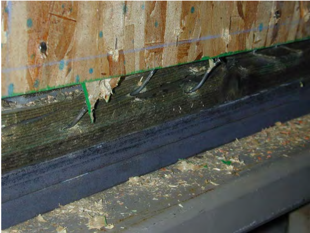
Figure 10. Fastener failure at sole plate, nail bending/ripping through sheathing (Specimen A3)
