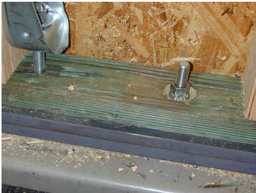
Figure 27. Anchor bolt showing slight embedment (but no bending) of washer (Specimen C3)
