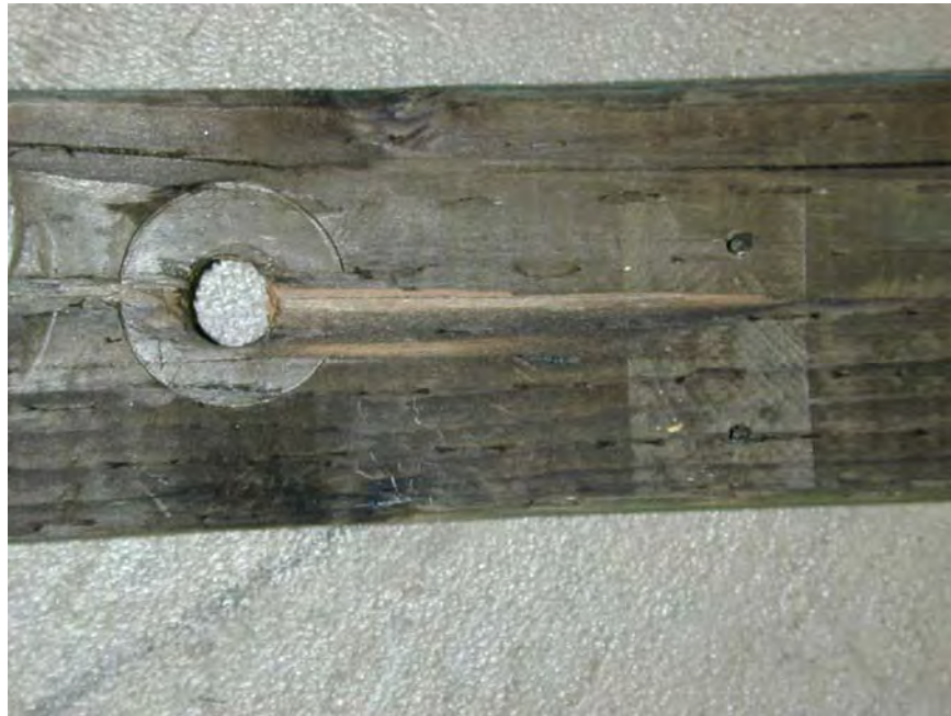
Figure 28. Sole plate (post-test) showing washer embedment (Specimen C2)
