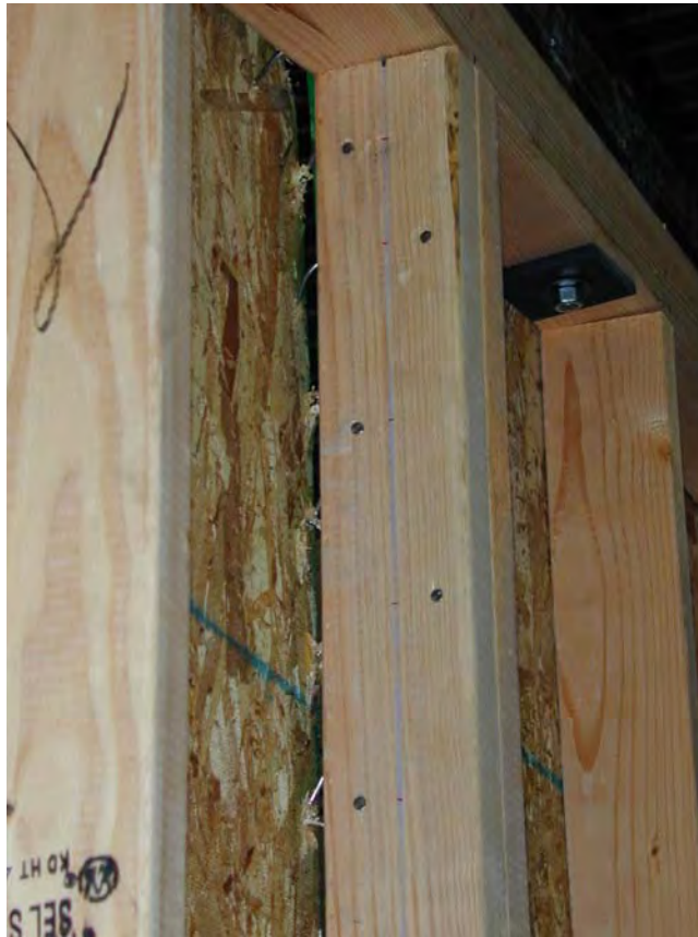
Figure 5. Fastener pull-out at panel edges along center stud (Specimen A1)
