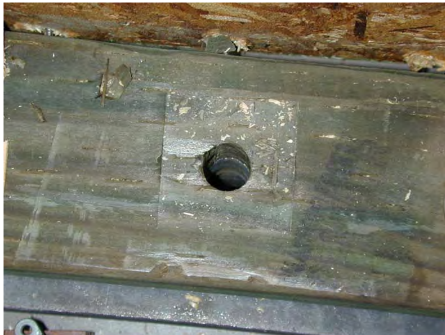
Figure 29. Sole plate (post-test) showing slight washer embedment (Specimen D2)
