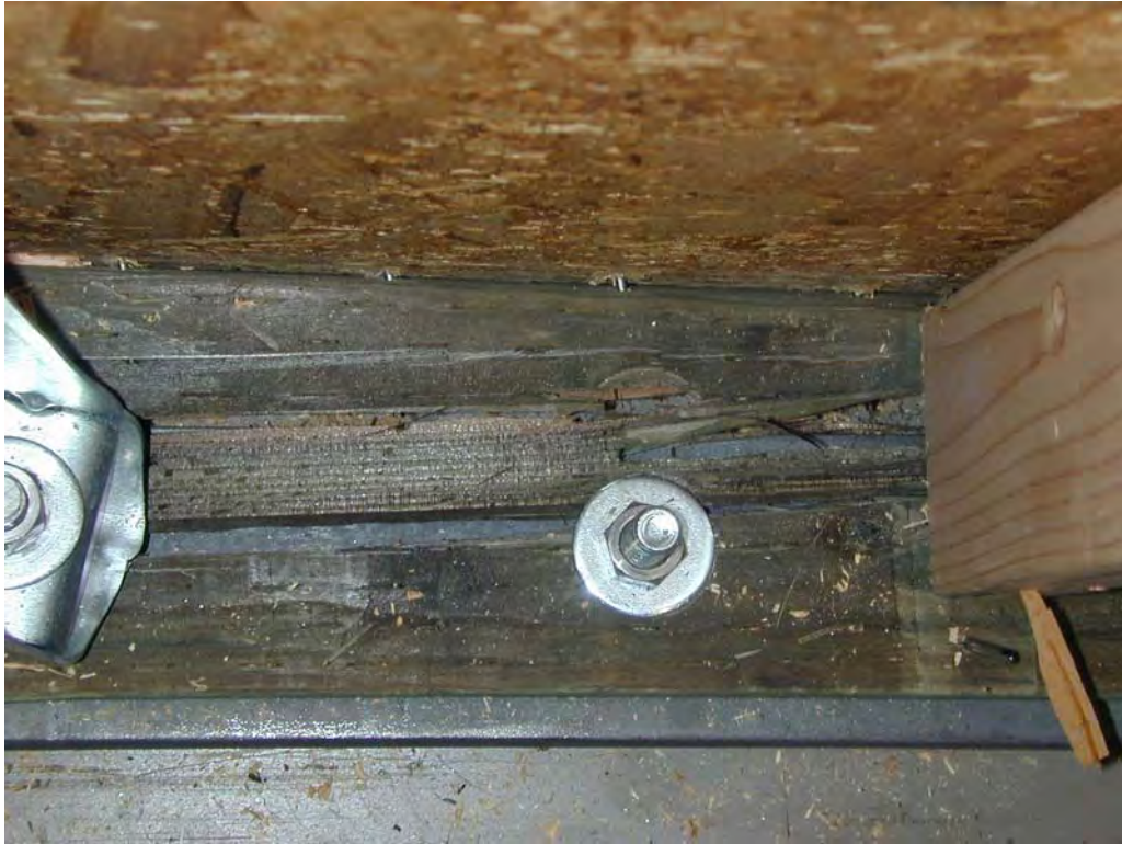
Figure 20. Top view of sole plate splitting from hold-down to first washer (Specimen C1)
