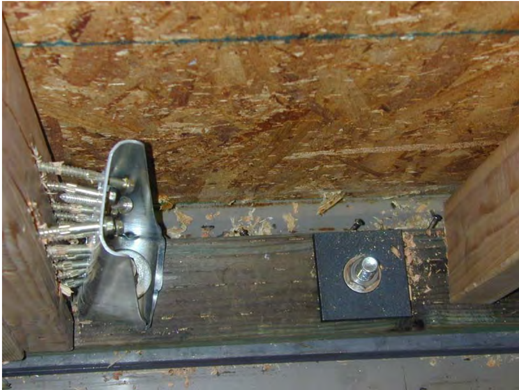
Figure 16. Multiple failures, but no splitting of sole plate (Specimen B1)
