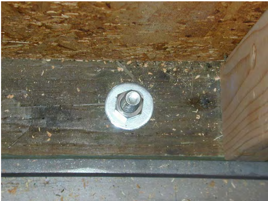
Figure 17. Start of a split in sole plate (Specimen C1)
