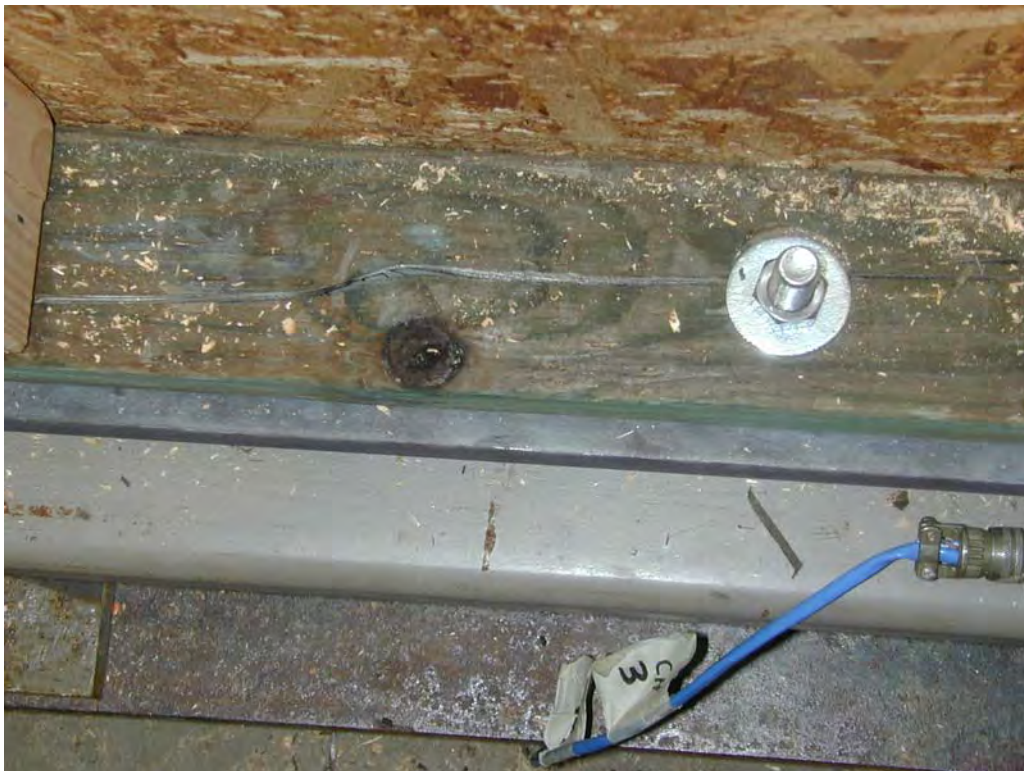
Figure 25. Sole plate split through interior bolt location (Specimen C1)
