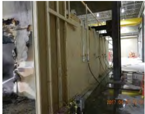
(b) exterior of exposed W1 after Test 1-5
