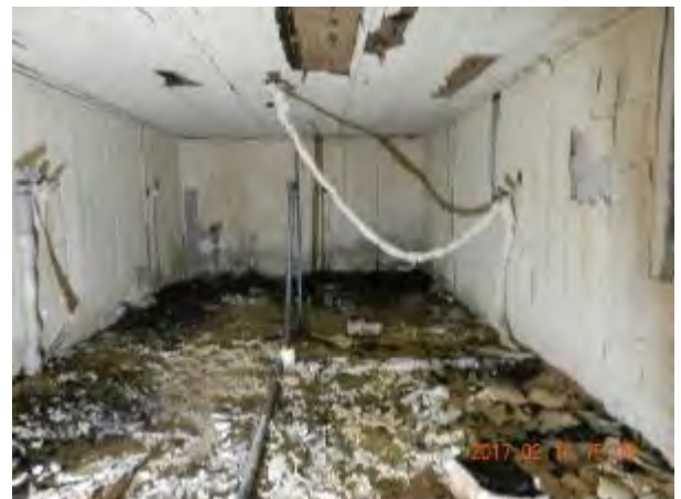
(f) after Test 1-1 – gypsum board remained: 2 layers on ceiling; 3 layers on walls
