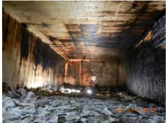
(b) W3, W4 W1 and ceiling CLT after Test 1-3.
