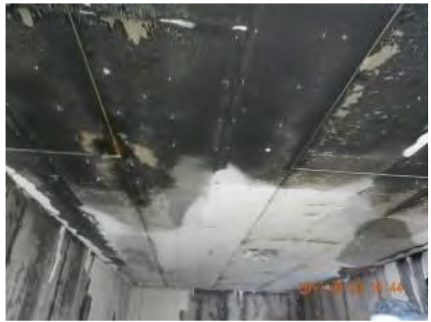
(f) after Test 1-2 – gypsum board remained: 1 layer on ceiling; 2 layers on walls
