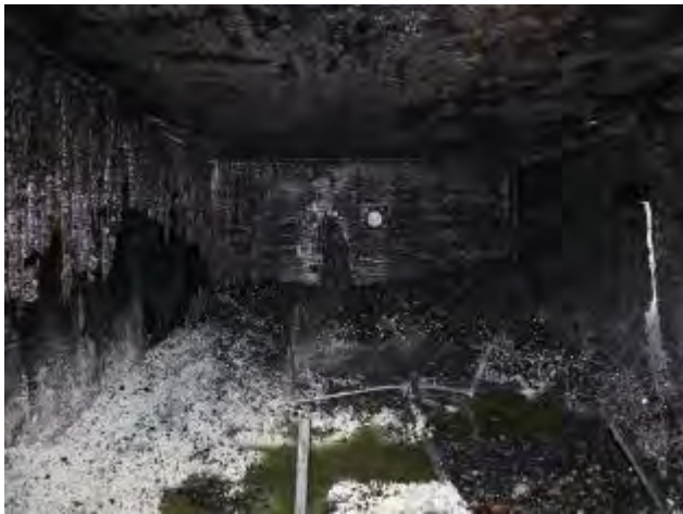
(a) interior of CLT compartment after Test 1-5
